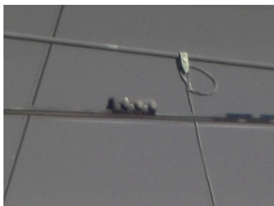
Contact wire splice
