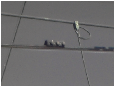
Contact wire splice
